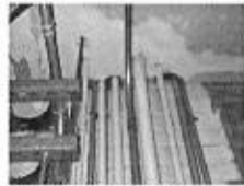
Boiler Room Pipe Penetrations
